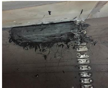
Rip repair beside bolt plate fasteners
